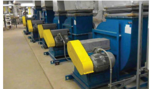
Figure 6: Installed on a VFD-controlled motor in an air handling unit at a community hospital in suburban Chicago, the AEGIS™ SGR Bearing Protection Ring reduced harmful shaft currents by 83% to levels well below those that damage bearings.
