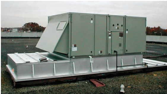
Figure 4: Rooftop HVAC unit in Michigan where a newly installed AEGIS™ SGR Bearing Protection Ring reduced shaft currents by 92% to levels well below those that damage bearings.
